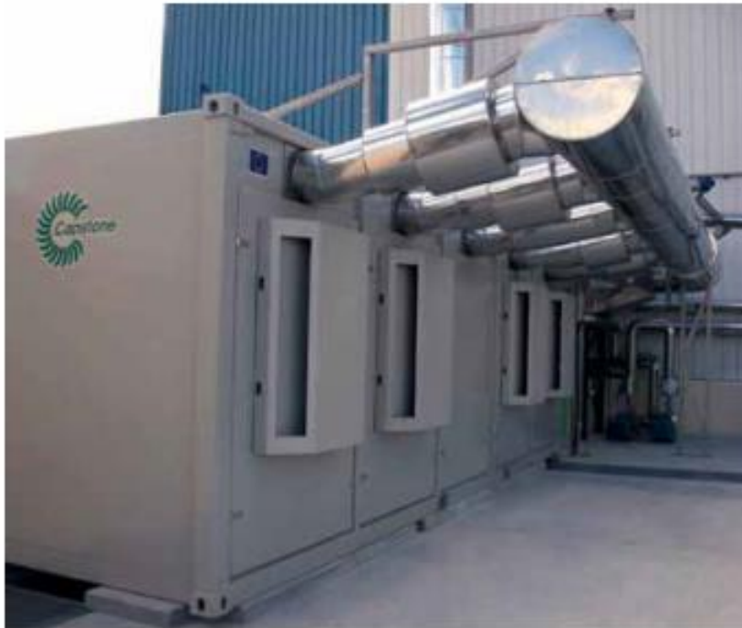
A C800 Power Package is fueled by methane from the treatment of sludge waste (from grape skins and stems) following the distillation of wine to make Cognac.
